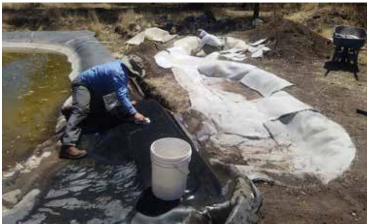
The construction of the main pond complete, lining and connecting the stream to the large pond.
