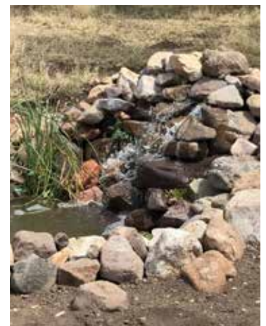
The completed flowing stream, with piled rock to allow for many microclimates to support Arizona treefrog.
