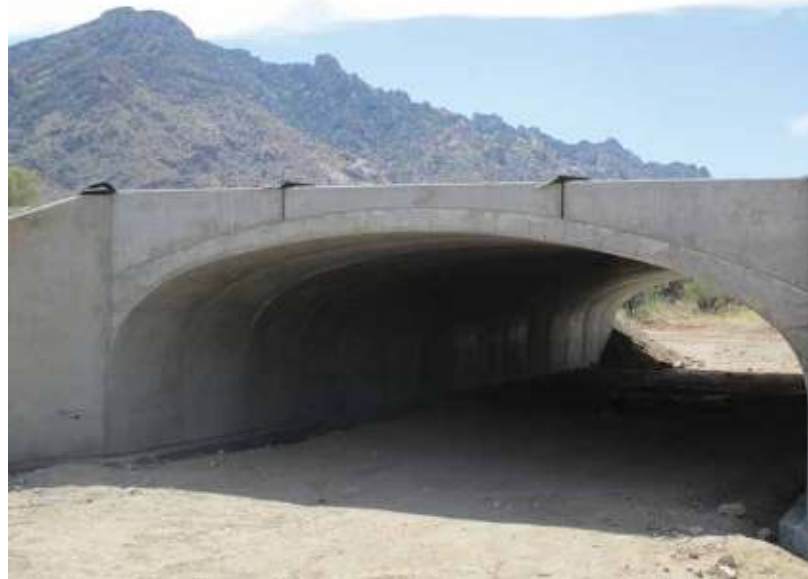
One of two wildlife crossing underpasses along State Route 86 on the Tohono O’odham Nation.
