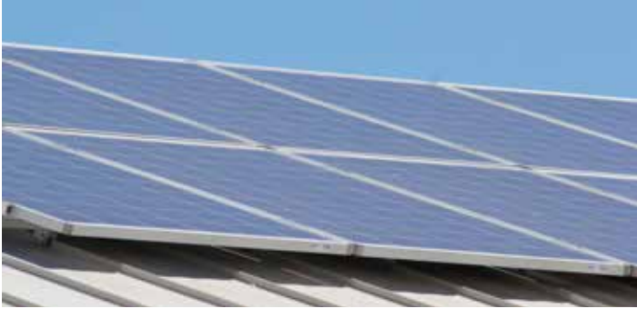
Some of the newer solar panels on the house roof
