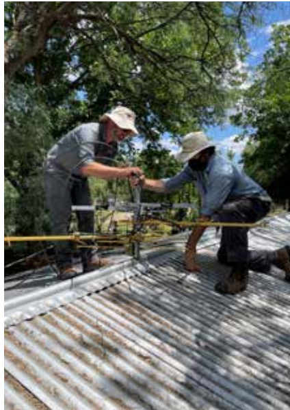
Our field crew installed the base for the antenna array to the casita at the Paton Center
